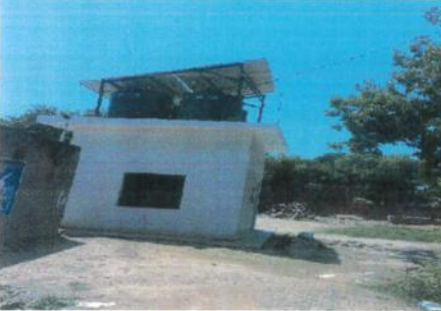
Solar Submersible pump room with storage tanks
